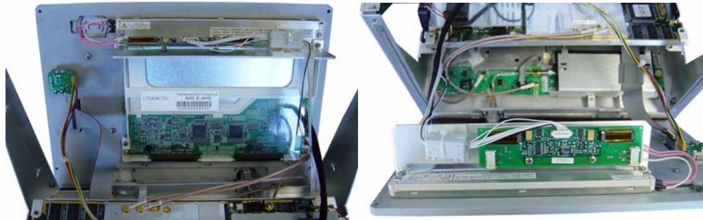
Figure 5-20. Front Panel Loose with Cables Attached
